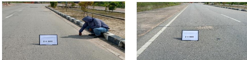
Figure 1. Road Damage Measurement at STA 2+500 – STA 2+600
