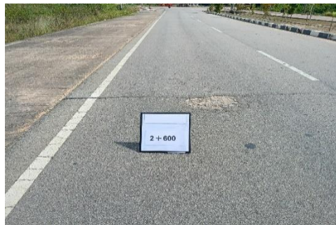
Figure 6. Transverse Crack Damage Of STA 2+500 - STA 2+600
