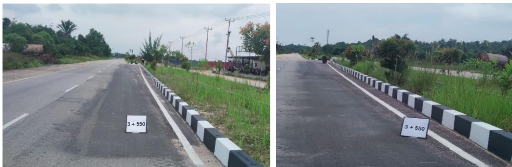
Figure 3. Road Damage Measurement at STA 3+450 – STA 3+550
