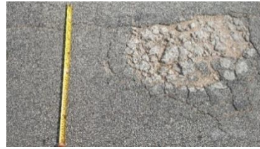
Figure 5. Pothole Damage on STA 2+500 - STA 2+600
